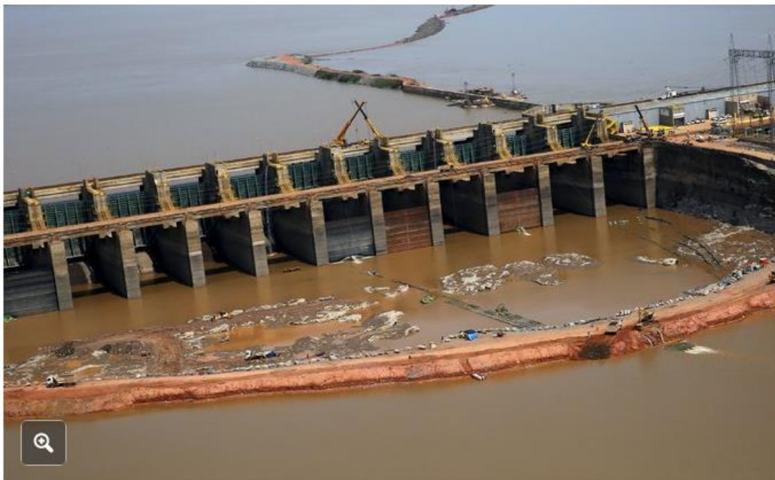
Construction of the Santo Antonio hydroelectric dam on the Madeira River in Porto Velho, Brazil. State-owned Chinese utilities have been investing in Brazil's economy. Nacho Doce/Reuters
